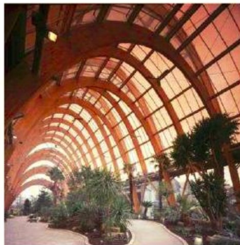
Figure 2: Sheffield Winter Gardens. The glulam arches for the roof were designed to EC 5 (TRADA, 2007).
