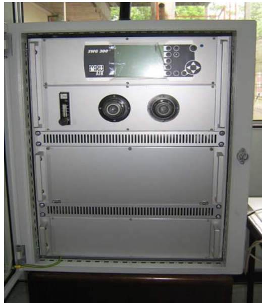
Figure 6-5: Flue gas analyzer, MRU
