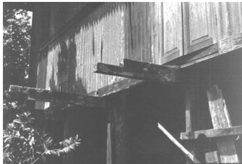
Fig. 10 – Floor beam projected out from Rumah Bujang indicates its connection with other parts of the house.
