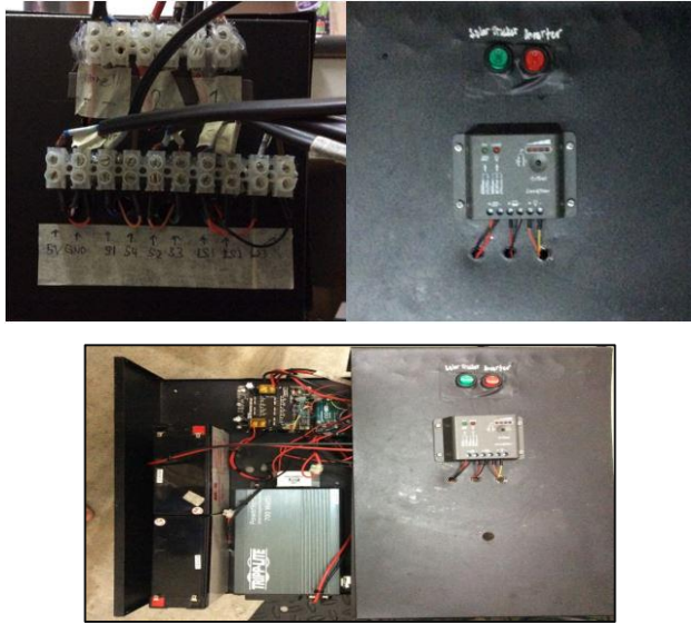
Figure 19 Controller Box Connection, Batteries, and Inverter
