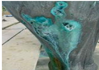
Zinc corrosion in sculpture
