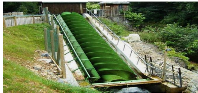
Figure 20 Archimedes Screw turbine (43)
