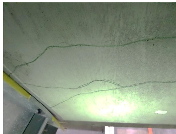
(b) Transverse cracks underneath slab M14 specimen
