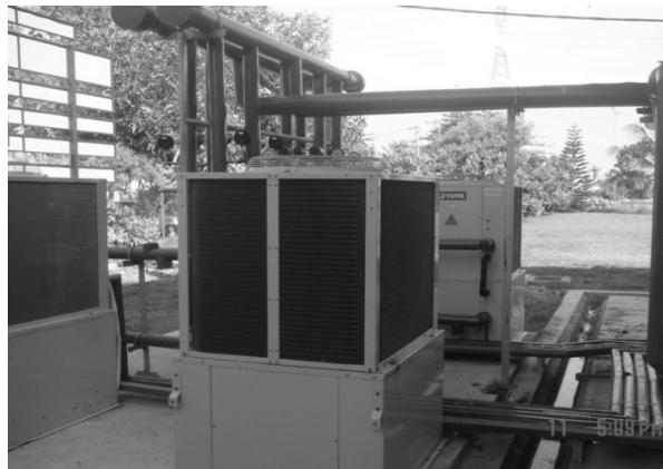
Figure 6. Air handling unit (AHU).
