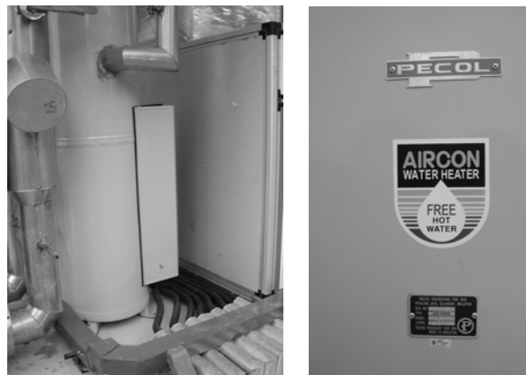
Figure 7. Heat recovery vessels.
