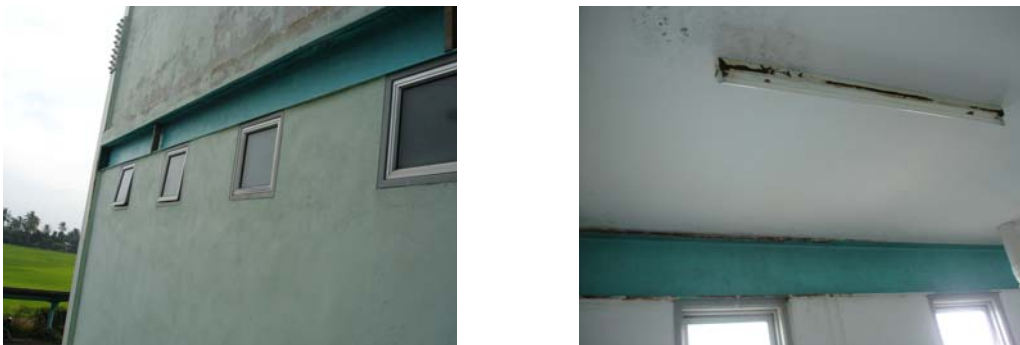
Figure 4 Steel beam should not be exposed to as in the case of concrete beam.
