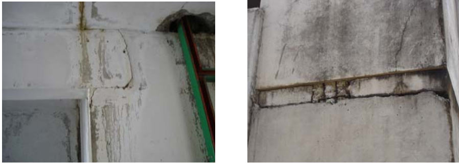
Figure 3 Poor connection system leads to issues of comfort and safety.
