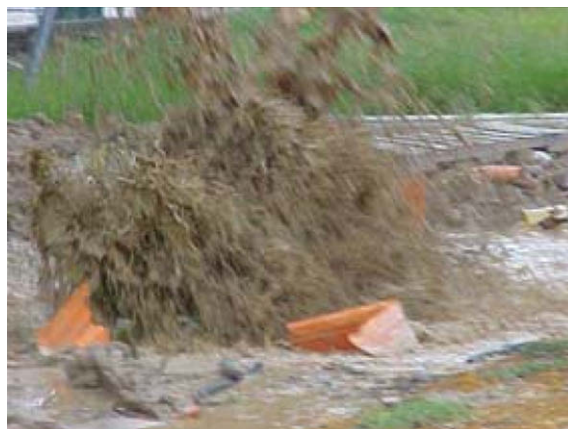
Fig. 1. Surface water splashing due to gas pipe leakages.
