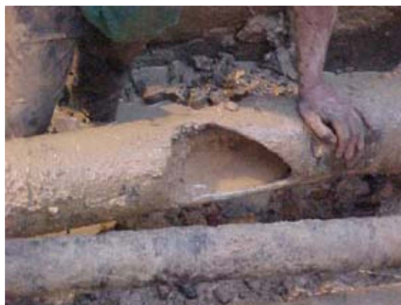
Fig. 14. Damaged asbestos pipe (water pipe).
