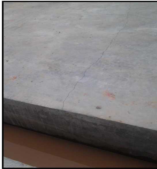
Figure 1.3: Crack on slab
