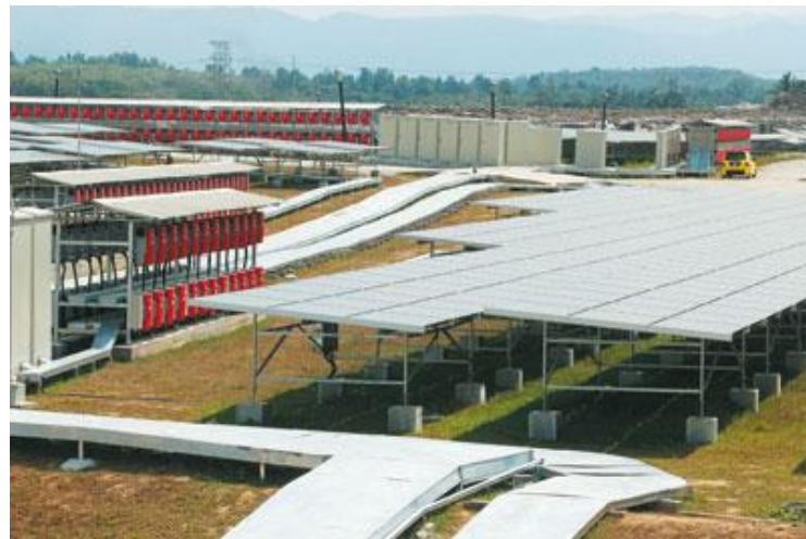
Figure 1.2 Cypark's 8MW solar farm, Negeri Sembilan
