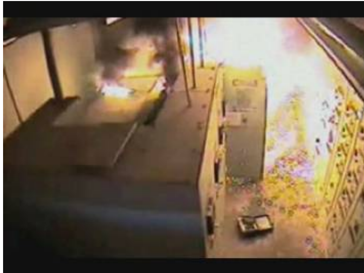
Figure 1.3 Arc flash from a switchgear panel
