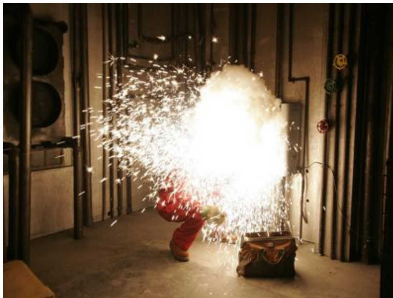
Figure 1.2 Arc flash generating a fire blast from a switchboard
