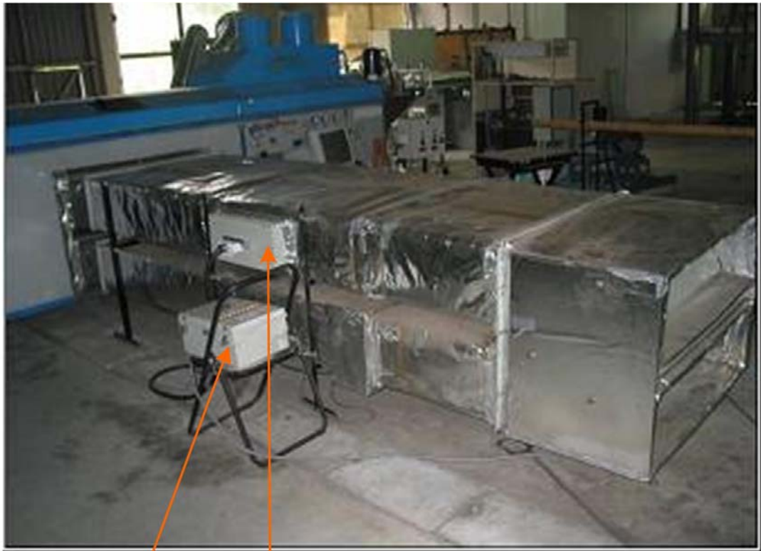
Heater controller ————— Electrical heater
