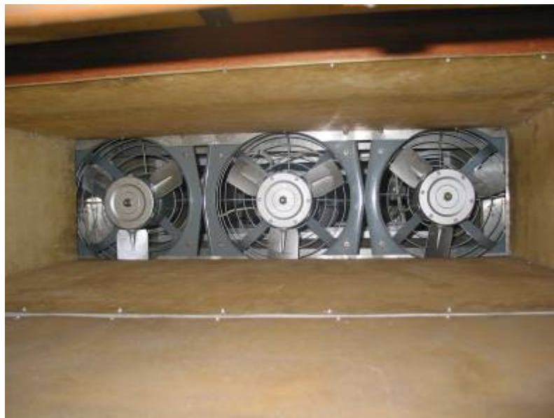
Figure H.14 Evaporator Auxiliary Exhaust Fan
