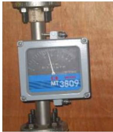
Figure I.6 Air Flow Meter
