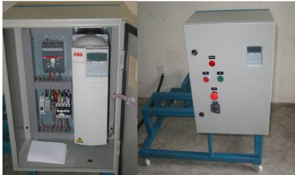
Figure H.5 Control Panel with ABB Inverter Attached
