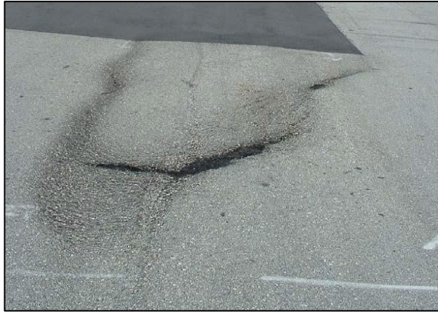
Figure 1.1: Slippage failure due to poor bonding between HMA layers (West et al, 2005)
