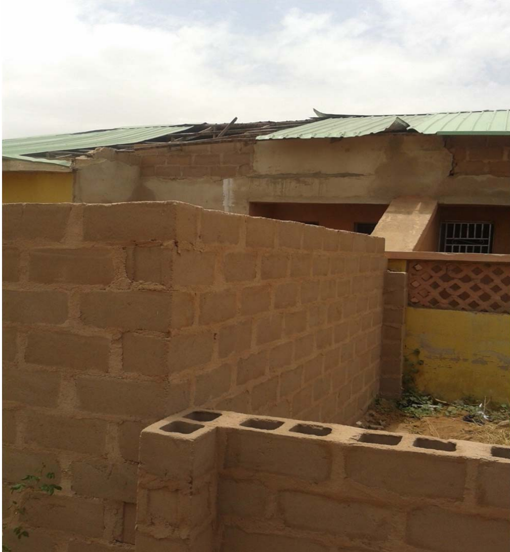
Figure 1.9: Illegal Building Extension due to lack of Monitoring and Control
