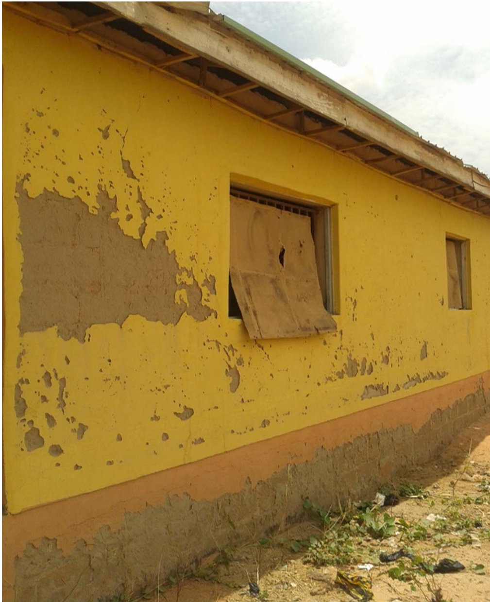
Figure 1.5: Exterior wall showing painting decay
