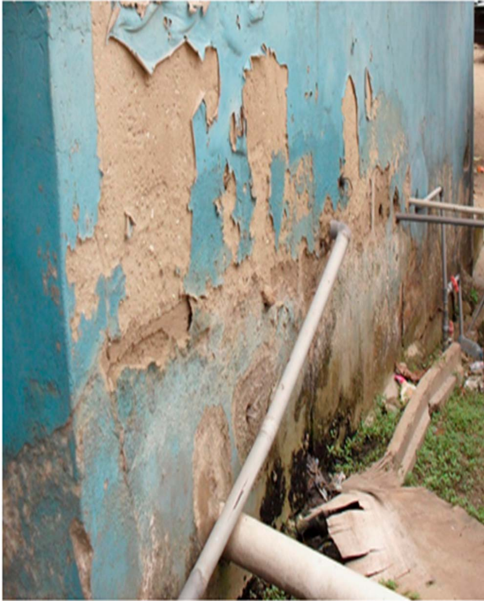
Figure 1.4: Exterior wall showing painting decay and poor plumbing work
