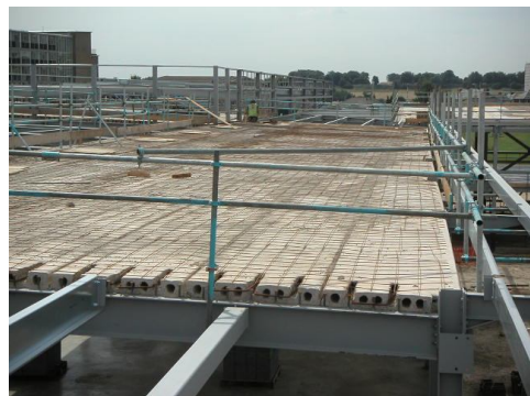
(b) Steel mesh are placed on to the precast slab before the casting of concrete topping
