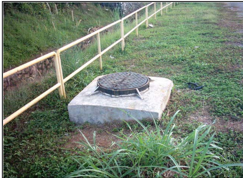
Figure 3.1: Abandoned Manhole (MH74a)
