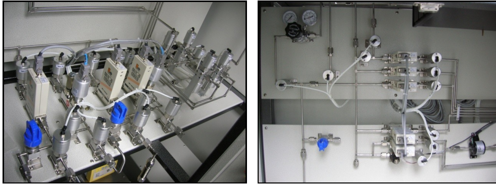
Figure 8 : MOCVD reactor delivery system with manifold gas panel.
