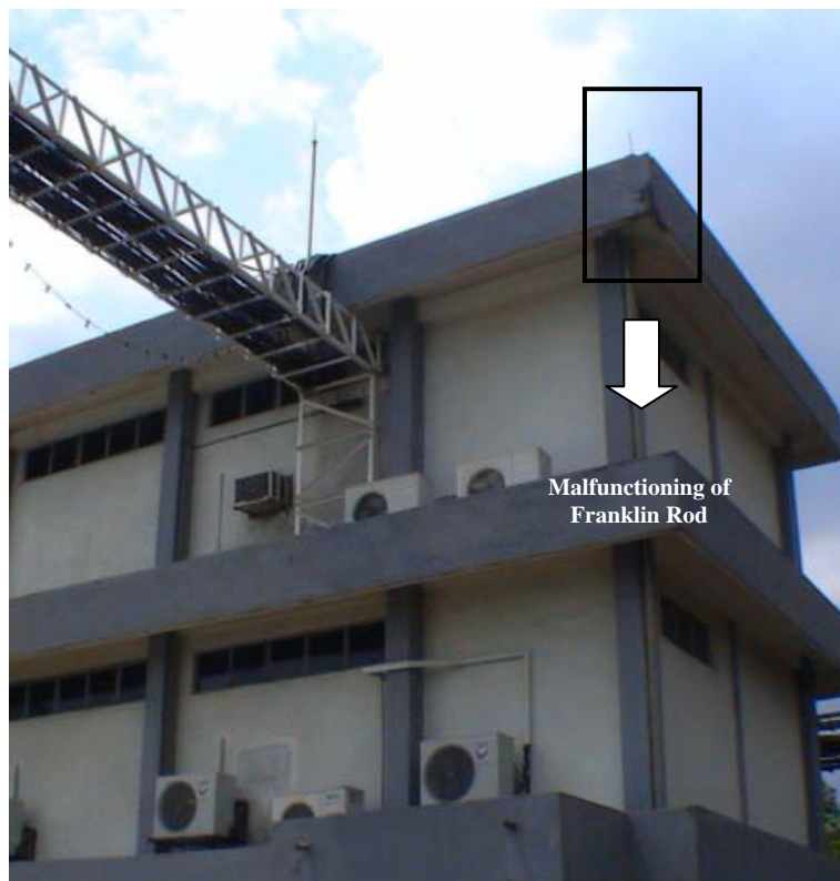
Figure 1. 2: Building structure equipped with a monopole at the roof top at the central and extreme edge of the building still being damaged by lightning stroke in spite of LAT installed.
