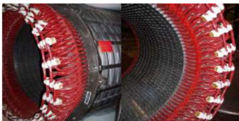
Figure 1. Winding of megawatt motor while the rotor removed.
