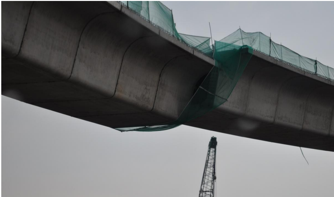
Figure 1.3 Misalignment of pre-cast box girder bridge near The New Istana Negara.
