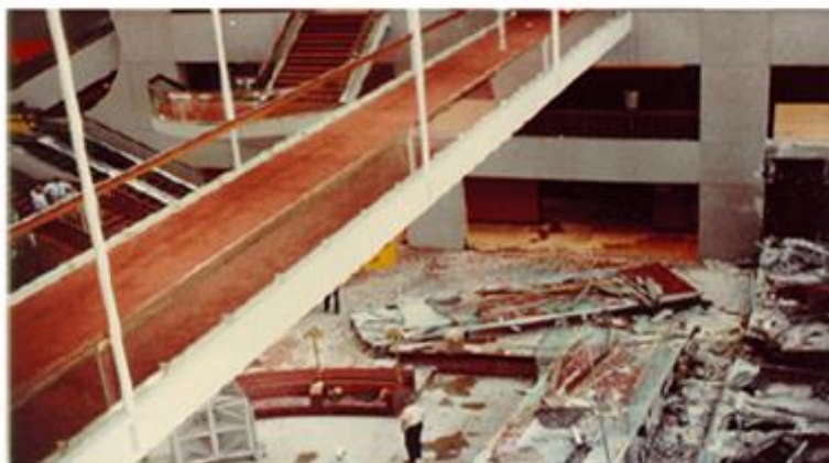
Figure 1.1 After Hyatt Regency Hotel walkway collapse in Kansas City in 1981 [1]
