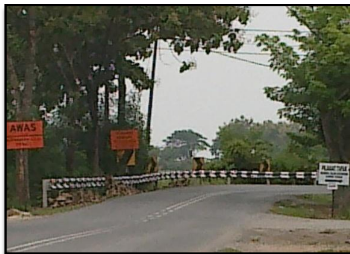
Figure 1.2: The second unsafe curve for the existing road
