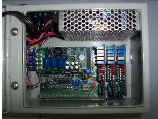
Figure 2.6: Inside view of FIU. FIU can add up to 4 cards (include main board) to monitor until 4 outputs feeder.
