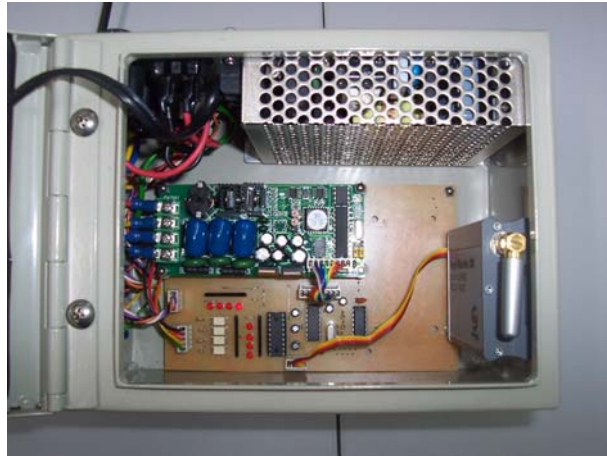
Figure 2.9: Inside view of FCU.
