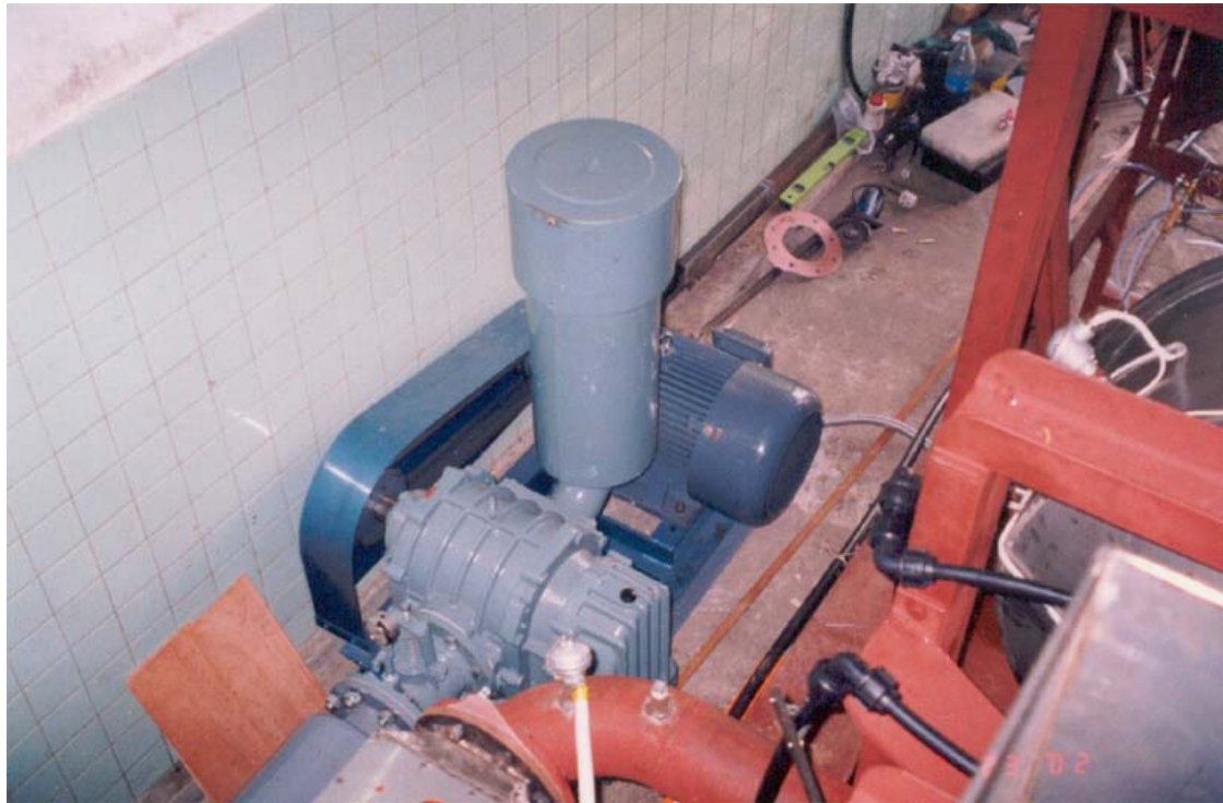
Plate 6.3: Primary blower unit
