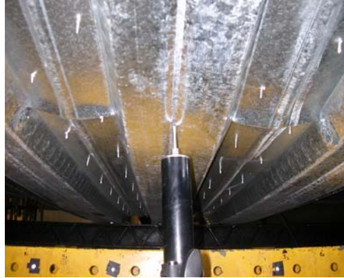
Fig. 8 Crippling of deck top flange and web
