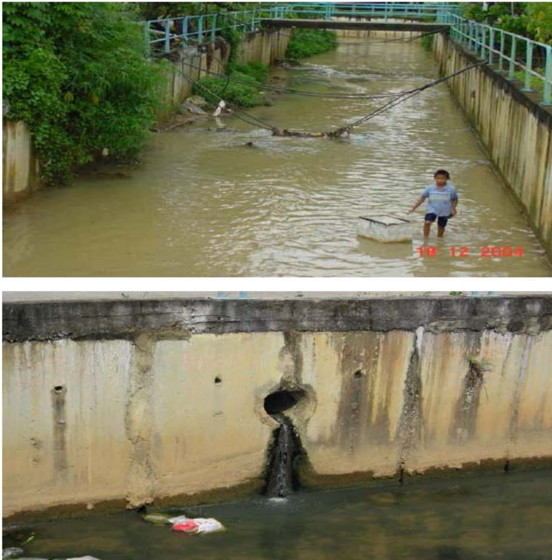
Figure 5.12: The condition of the concrete channel in year 2004.
