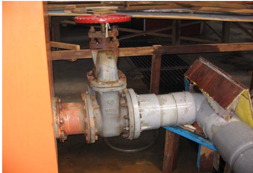
Figure 3.4 Valve in front of flume
