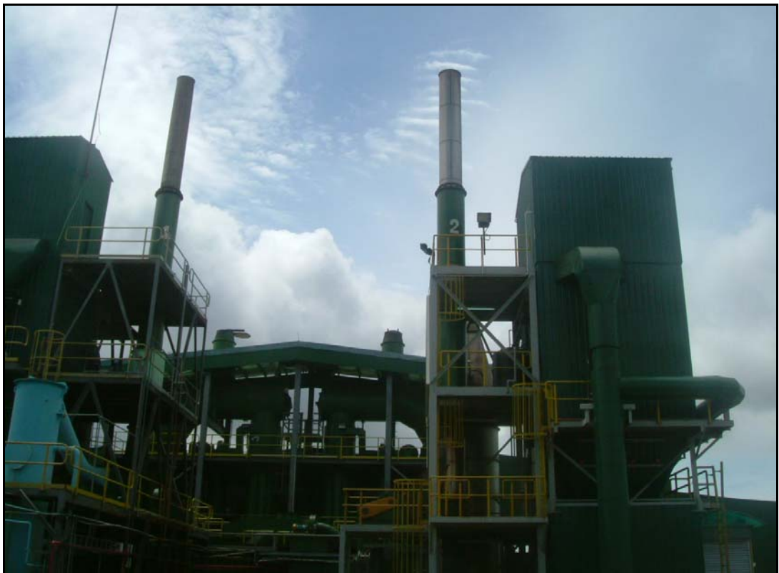
Figure 2.3 The Incineration Plant owned by Pantai Medinvest Sdn Bhd. in Malacca
