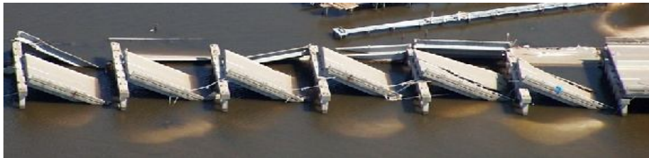
Figure 1.2 Unseating of the bridge deck of Shoowa Bridge in 1964 Niigata earthquake (Moehle and Eberhad, 2000)
