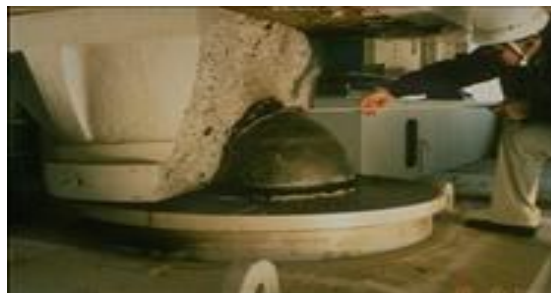
Figure 1.3 Nishinomiya-ko Bridge bearing failure in 1995 (Moehle and Eberhad, 2000)
