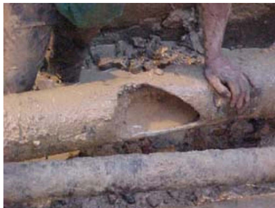
Fig. 14. Damaged asbestos pipe (water pipe).
