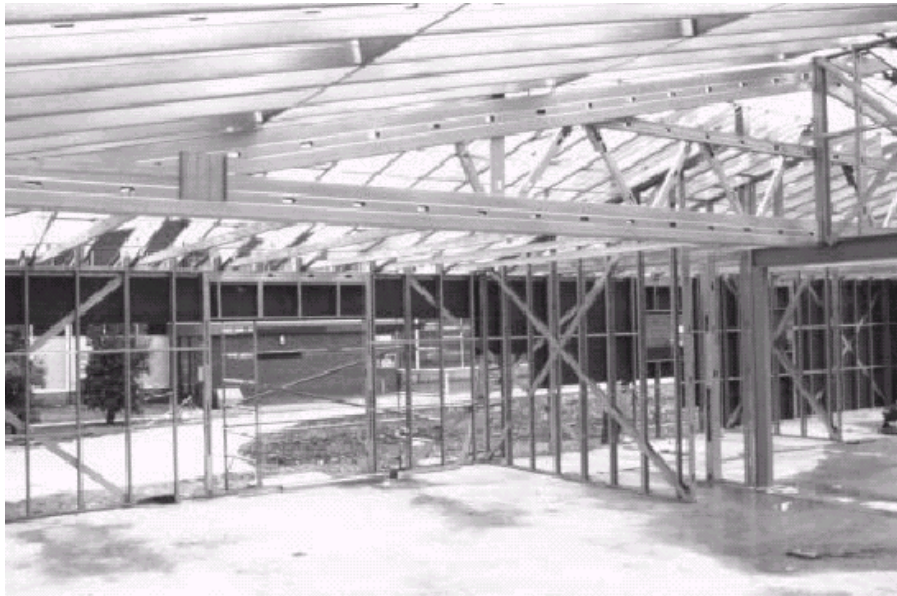
Figure 1.3: Cold-formed light steel framing for residential house (adopted from Lawson et al. , 2002)
