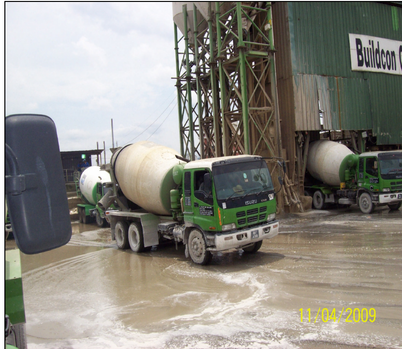
Figure 1.2 : Concrete batching plant
