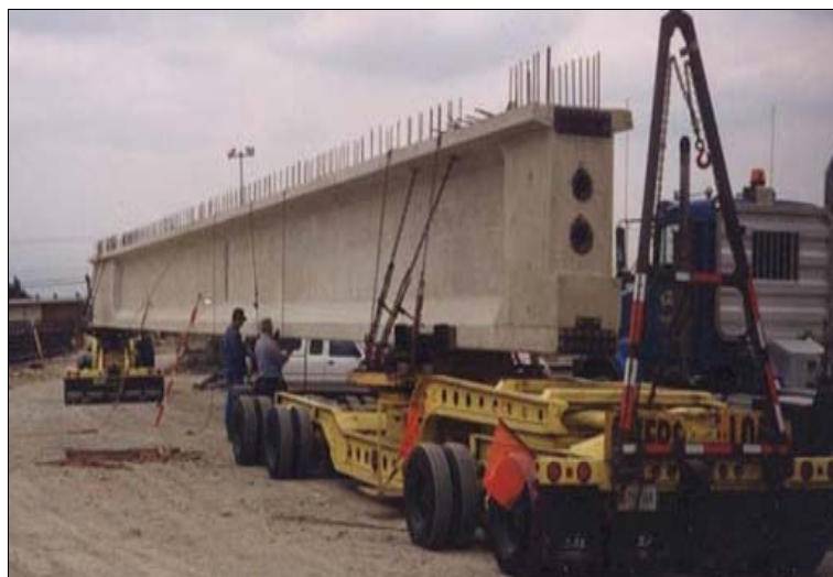
Figure 1.1: Length and weight limits on precast beams lead to splicing for longer spans
