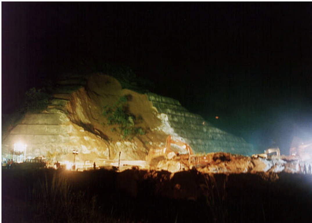
Figure 1.1 View of slope failure at KM303 NB, Section C1, NSE
