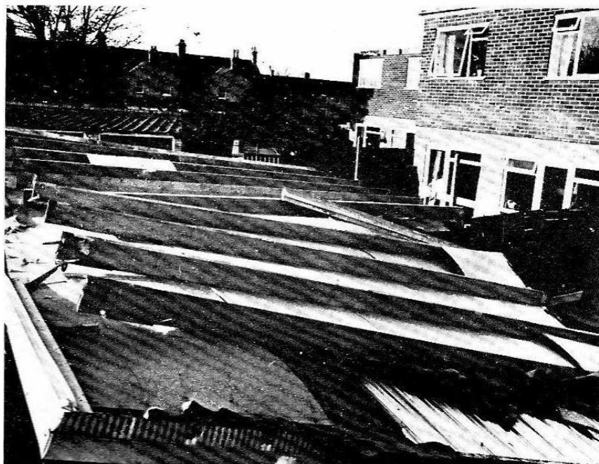
Figure 1.1: Some of the common example of roof failure
