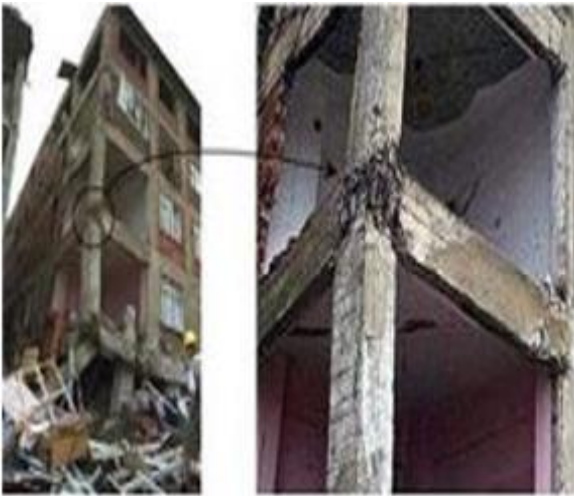
Figure 1a Joint Failure
