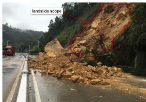
Figure 8. S203 line landslide site.
