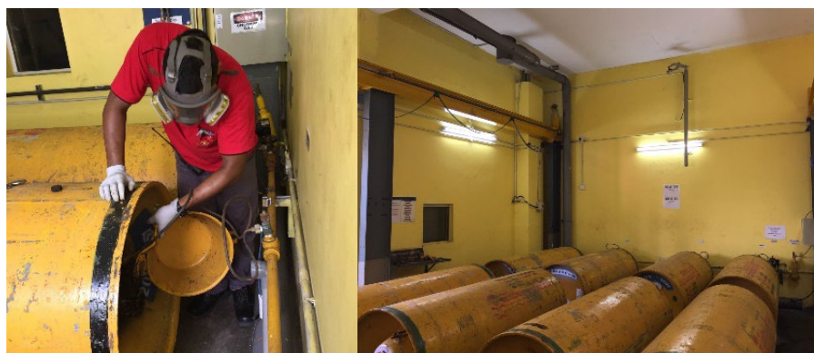
Figure 3. Chlorine room and drum replacement in progress.
