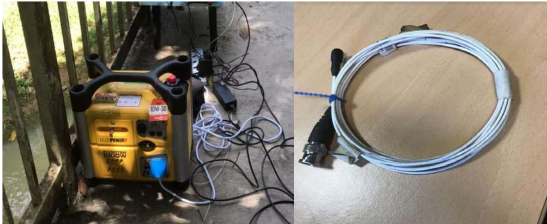
Figure 7a. 800-watt portable generator for power supply
