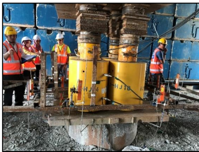
Figure 7. Load cells and pressure gauges
