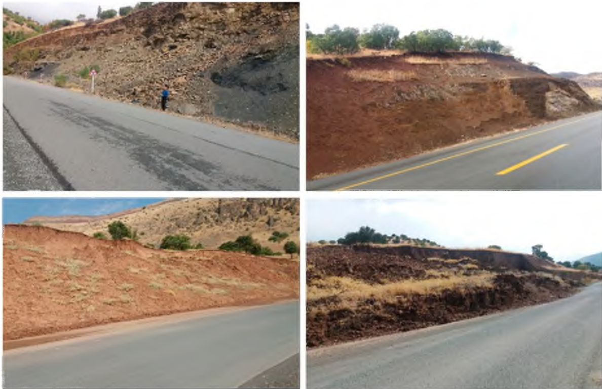
Figure 3. Examples of landslides located along the Kamyaran–Sarvabad main road, Iran.
