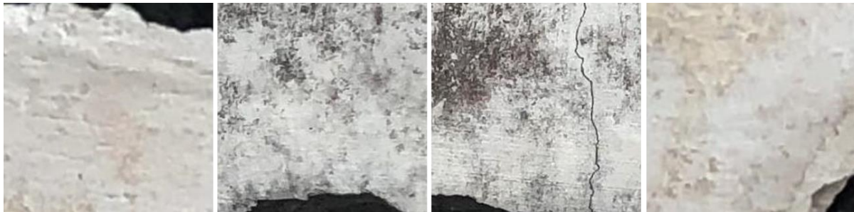
Fig. 5. Presence of cracks on the edges of testing cropped image spaces
