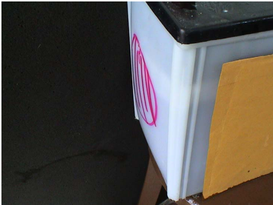
Figure 4 : Typical problems on maintenance free battery (bulged/ swollen)
