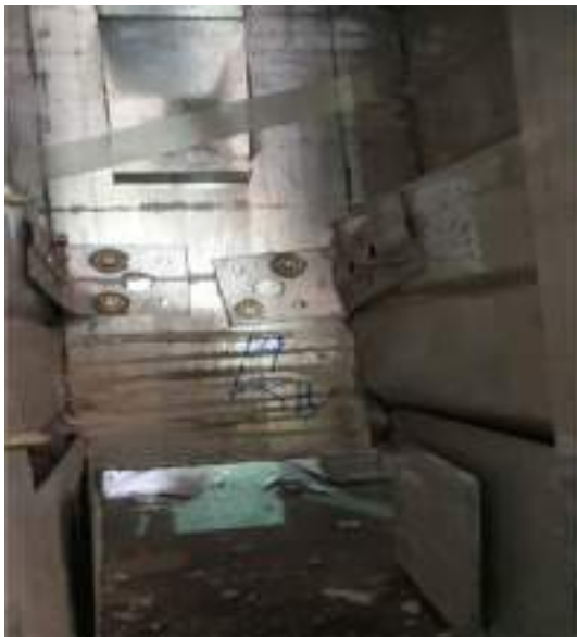
Fig. 40 Buckling of the brackets holding the concrete slab
