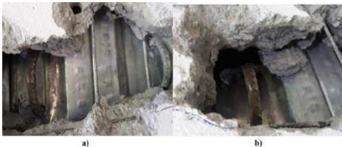
Fig. 51 Shear connector status after the test
