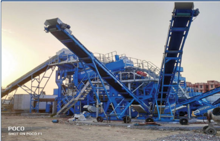
Fig. 4 Photograph of wet proccession unit at New Delhi, India
