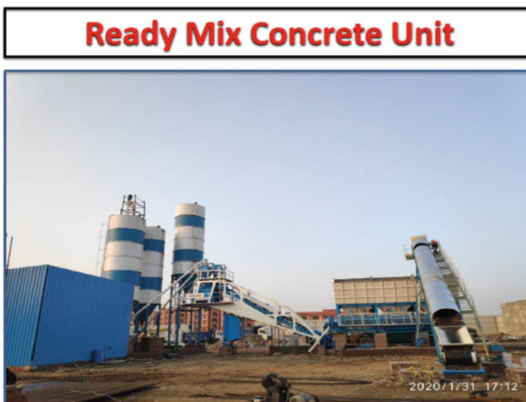
Fig. 6 Photograph showing Ready Mixed Concrete Unit
