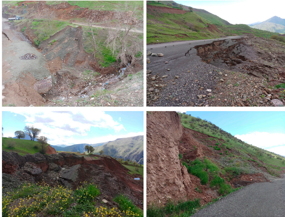
FIGURE 2 | The photographs of the landslides occurred in the study area.
