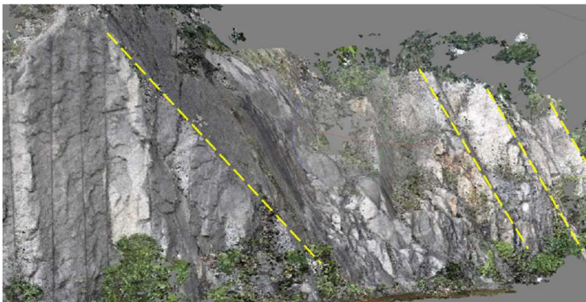
FIGURE 4. The point cloud model obtained from photogrammetry survey of Slope KSA, showing signs of relic planar failure as shown in yellow dashed lines
