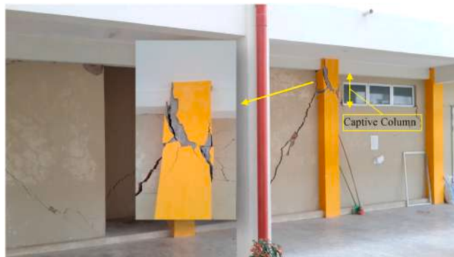
Fig. 1. Shear failure of a captive column during 2015 Sabah earthquake, Malaysia [2].
