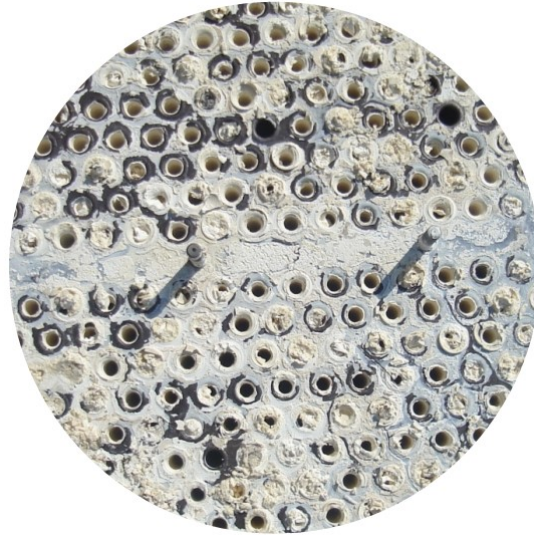
Figure 1.1: A cross-sectional view of heat exchanger shows severe deposits [19]
